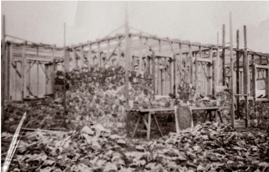
26 Pioneer Drive, took three winters to build, during the off honey season
